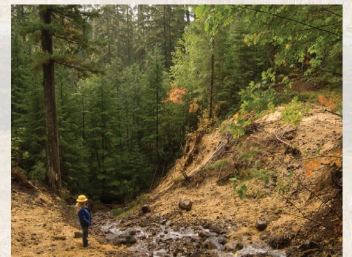
South Fork road decommissioning, after stream crossing restoration at culvert, and road fill removal. Photo credit: Robert Metzger, US Forest Service
