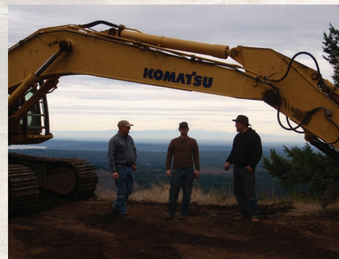
2013 North Fork Skokomish road decommissioning. Photo credit: Robert Metzger, US Forest Service
