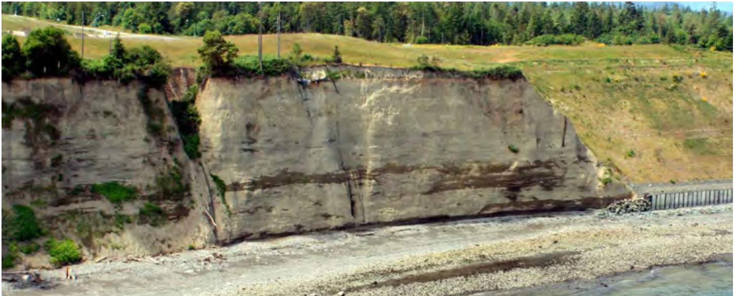
Active bluff on east cell 304 and beginning of seawall at west cell 304
