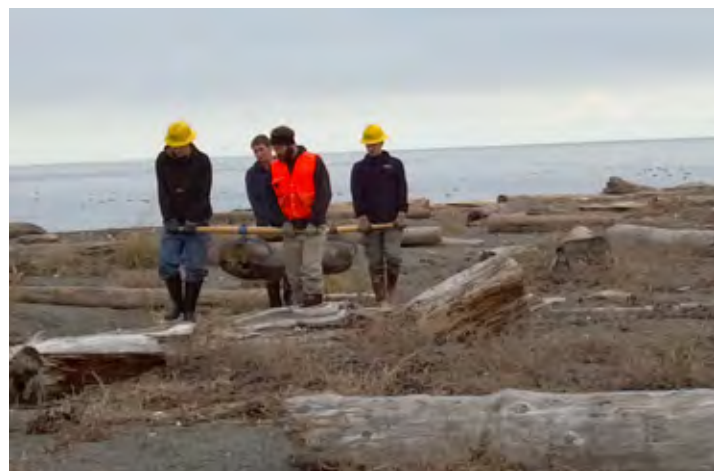
Washington Conservation Corps crew removing beached creosote-contaminated wood at 3 Crabs Beach, Clallam County
