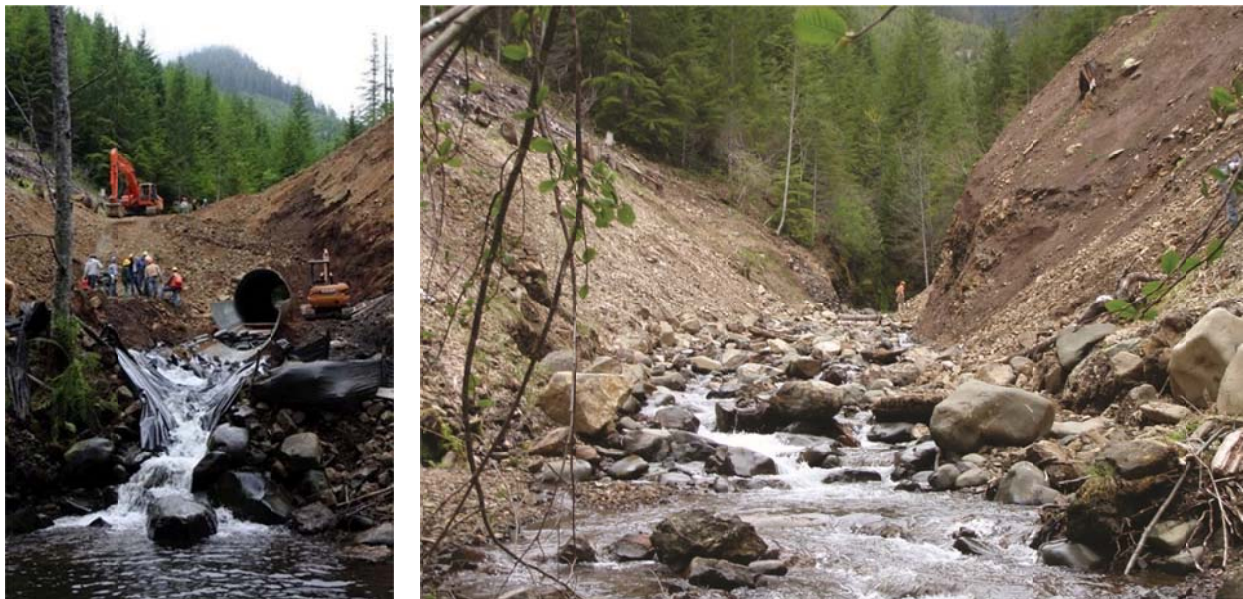
Figure 4-1. An example of culvert and road fill removal on a tributary drainage to the upper South Fork (USFS 2017).
